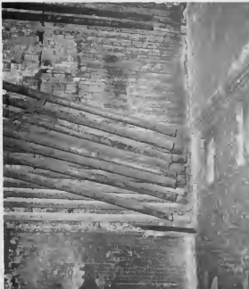
THE INSIDE of the furnace on No. 9 Visbreaker looks like this before the back brick wall is dismantled. Pipes in the convection section hang down just before being pulled. A new wall with bracing will replace the back wall. A bulldozer operator, right, watches out a tube handle with the help of a derrick, not shown.
